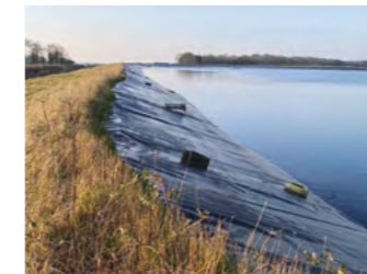
2. HDPE membrane lined reservoir
